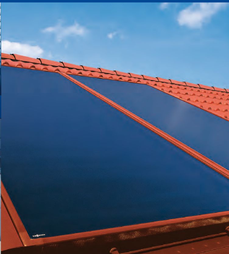
Thermal insulation of solar collectors, Viessmann, D
